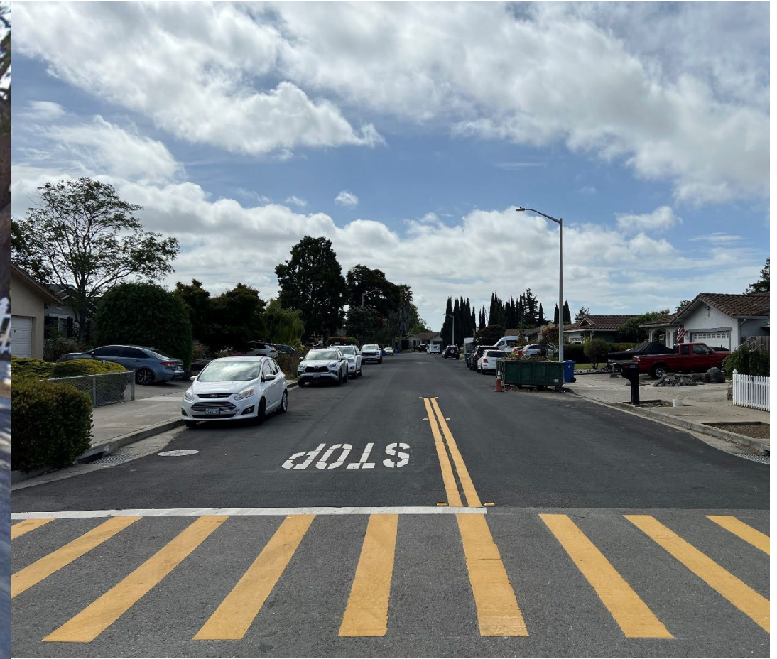
Figure 12: Jacaranda Drive After Patch Paving, Application of Rubberized Cape Seal, New Striping, New High Visibility Continental Crosswalk
