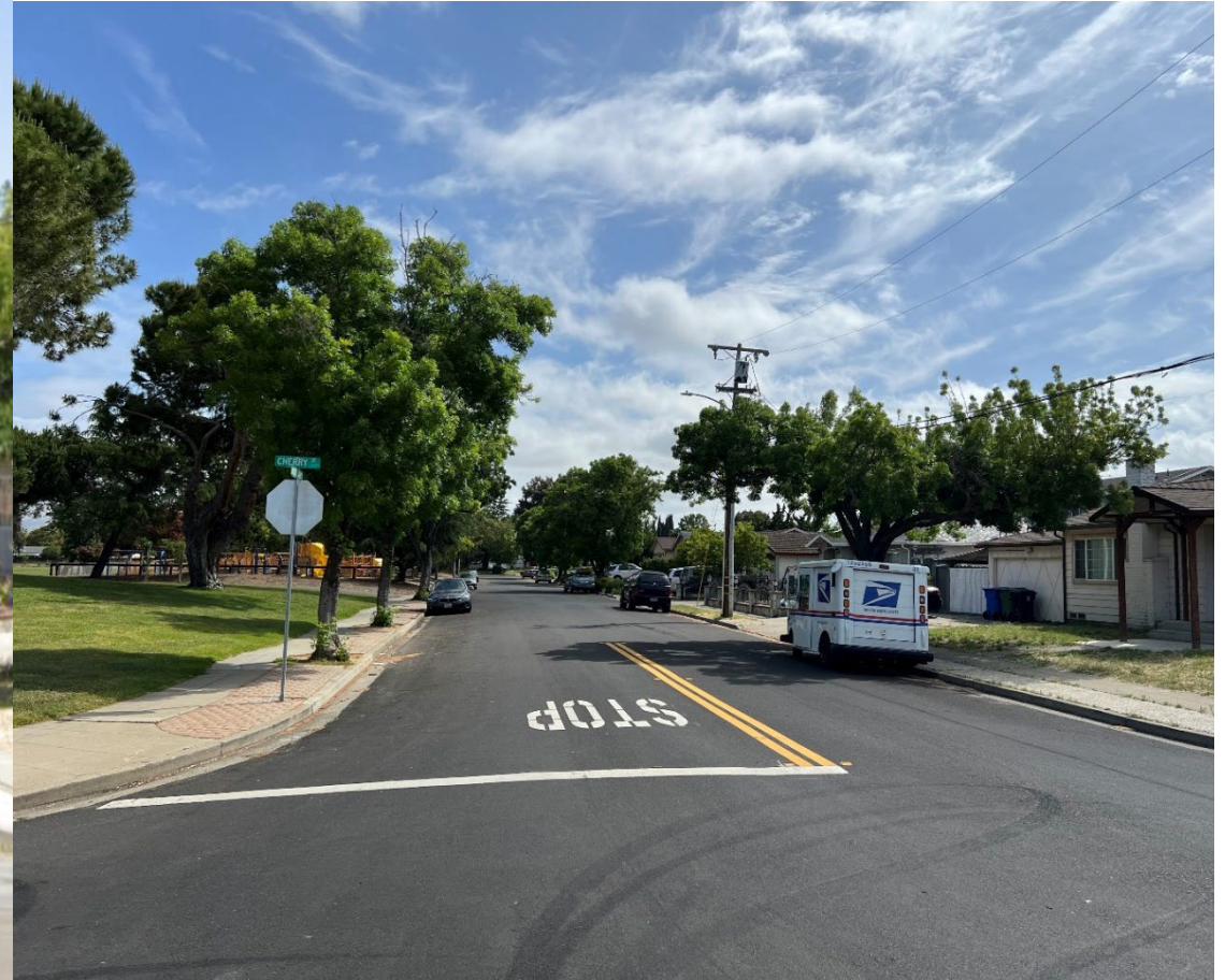
Figure 14: Montcalm Avenue After Patch Paving, Application of Rubberized Cape Seal, and New Striping
