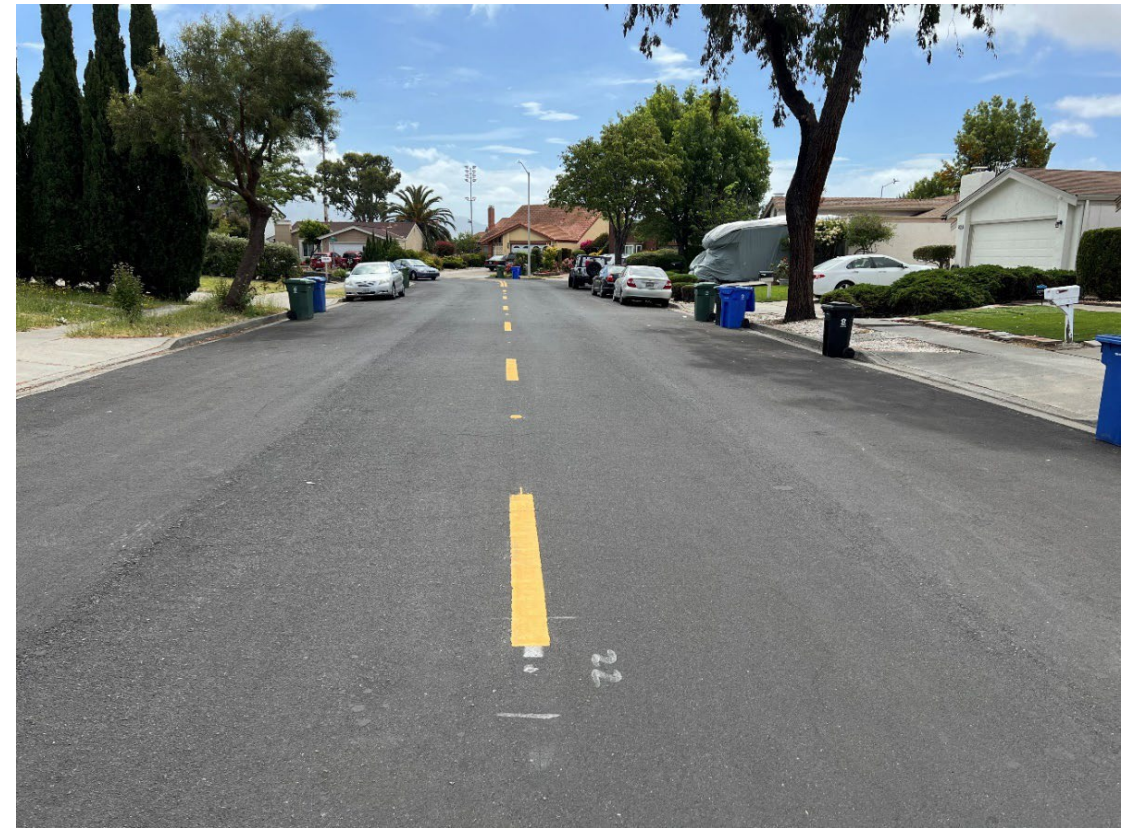
Figure 16: Ebbetts Street After Patch Paving, Application of Rubberized Cape Seal, and New Striping
