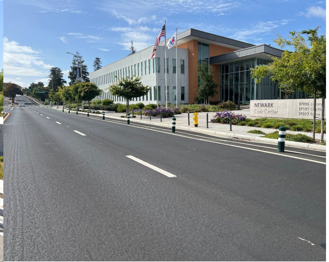
Figure 4: Newark Boulevard in Front of City Hall and Library After Patch Paving, Application of Slurry Seal, New Lane Striping, and Class IV Separated Bikeway
