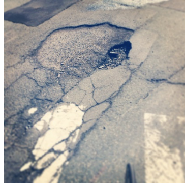
Poor pavement quality ahead of a bike lane
