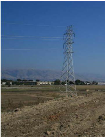
PG&E high voltage tower within Area Two.
