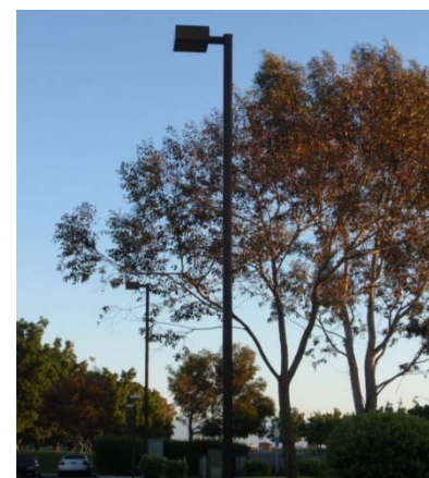
Figure 4.7: Outdoor parking lights
