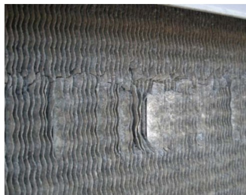
Figure 4.13 – Carrier Coil Deterioration
