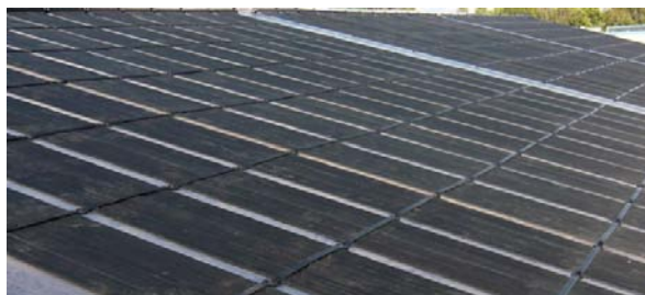
Figure 4.4 Solar Thermal Installation (typical)
