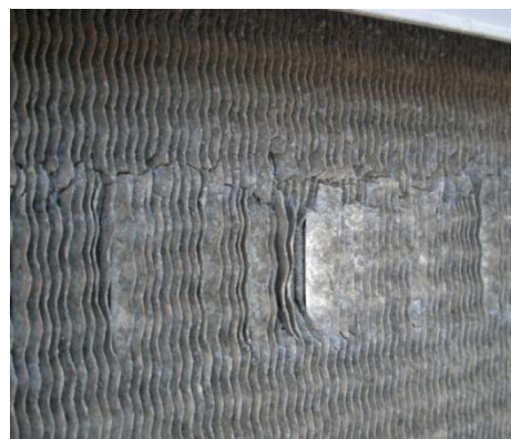
Figure 2.2: Gymnasium Unit Coils
