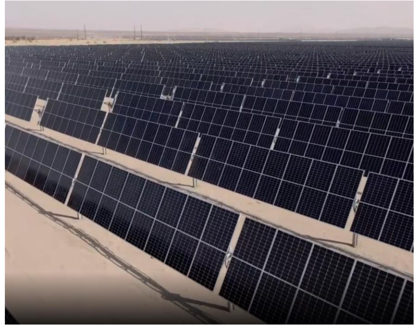
Rosamond Central Solar Project | Commissioned in December 2020
